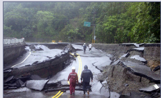
Road damaged by Typhoon Morakot in 2009. Source: CNN.
